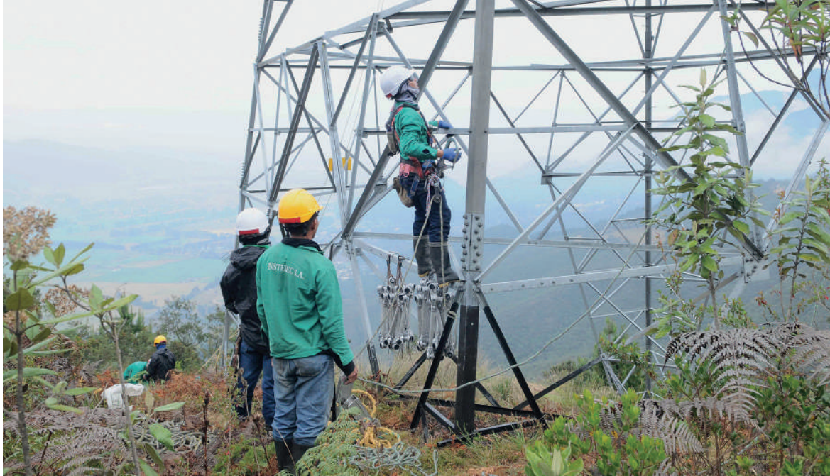
Raising of transmission tower at the 309 project in Pradera (Valle), Tesalia - Alférez Project
